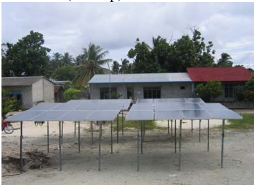
FIGURE 13: Solar PV System installed in B. Goidhoo and R. Fainu (8 kWp)
