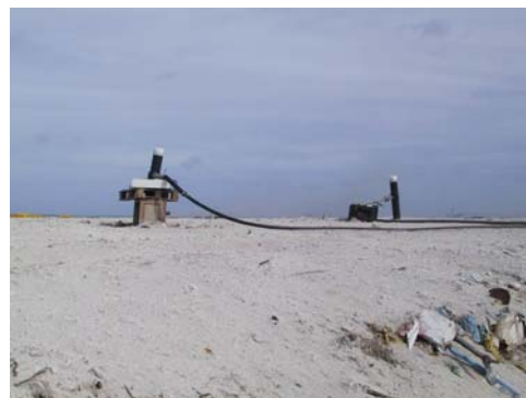
FIGURE 18: Landfill gas recovery plant
