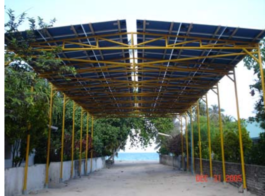
FIGURE 12: Solar-Diesel Hybrid System installed in Adh. Mandhoo
