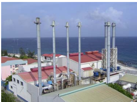
FIGURE 3: STELCO Power Plant in Male', (Source: MEEW)
